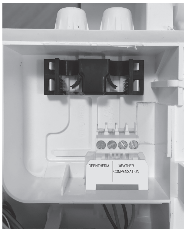
INSTALLER CONNECTIONS (RHS)
